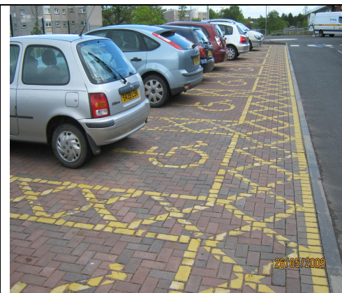
Photo 7. Permeable paving at disabled parking spaces
