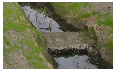
Check Dam to control flow velocity
