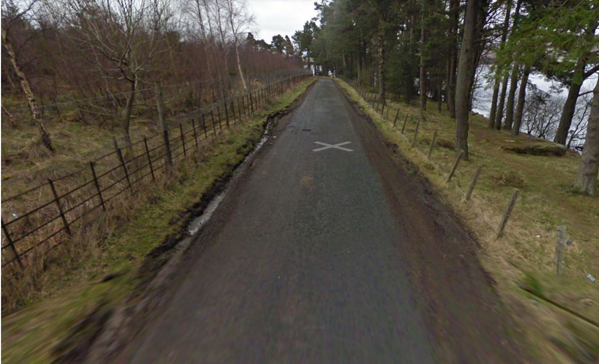
Figure 1 Damaged grass verges due to parking (Source: Google)
