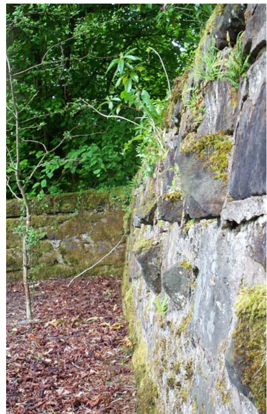
Defective cement pointing in rubble walls
