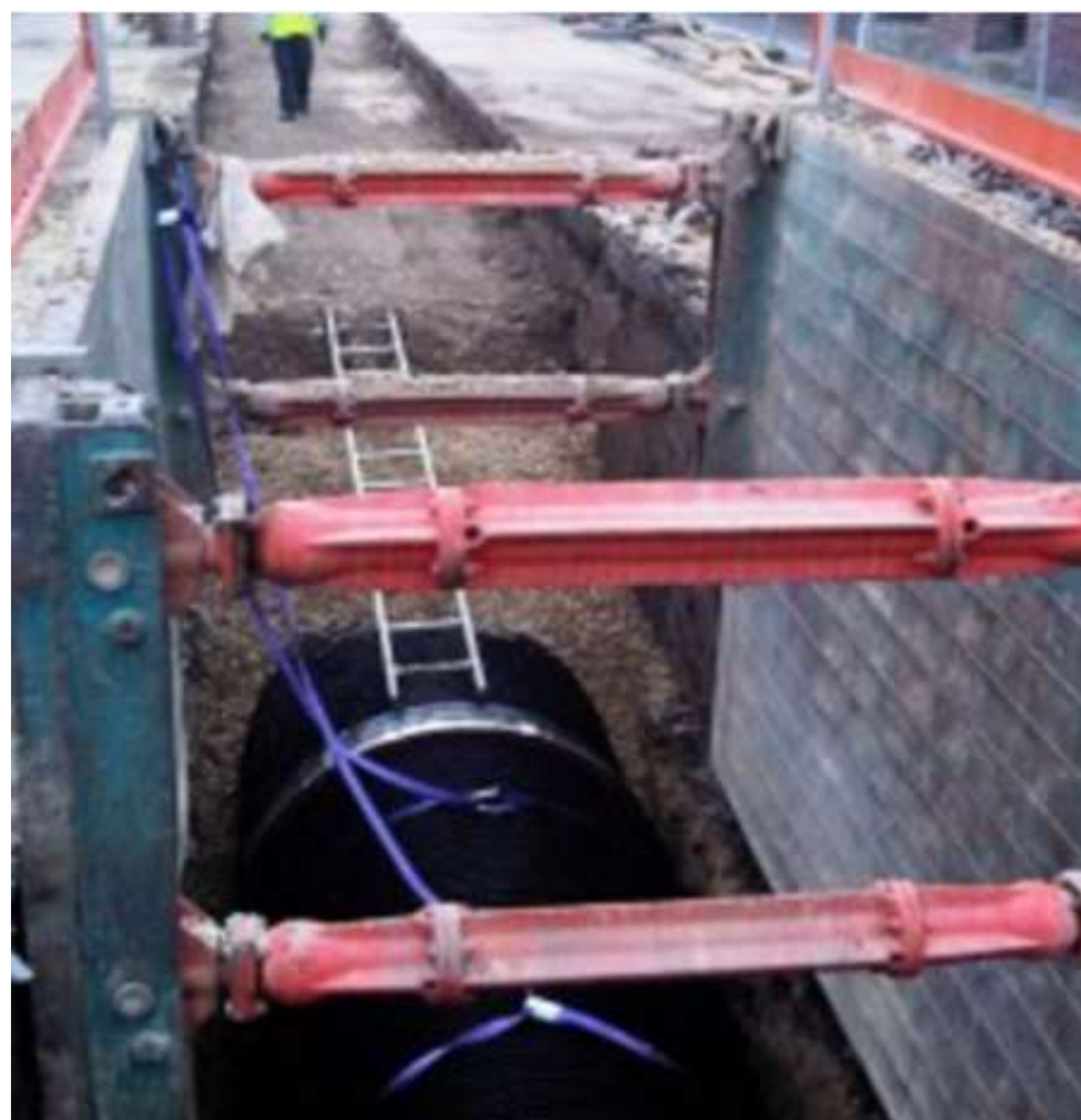
Example of excavation and trench supports for installation of a large diameter trunk sewer.
